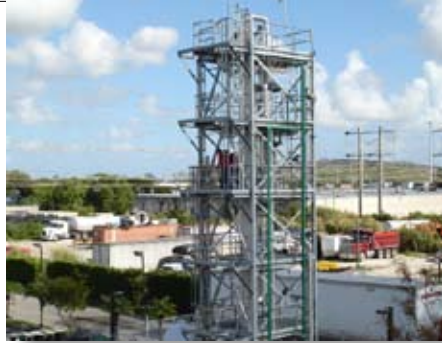
Distillation system at a wastewater treatment facility
